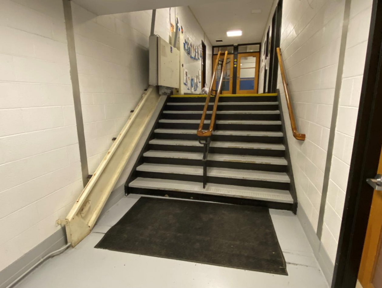
Lift at Stair
