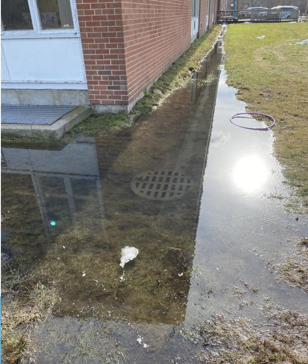
Clogged site drains, poor soil drainage
