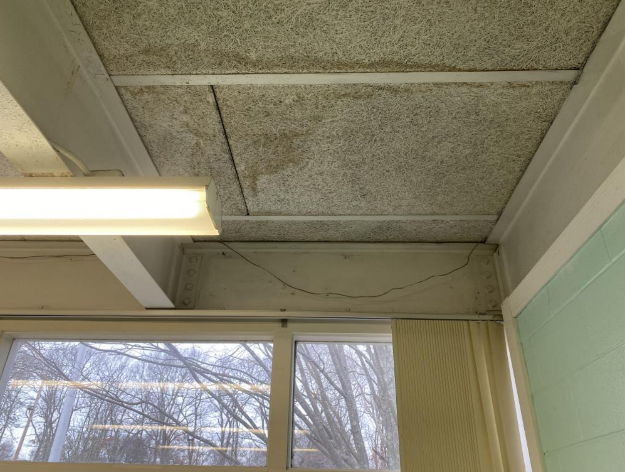
Roof leaks, roof decking not easily repairable
