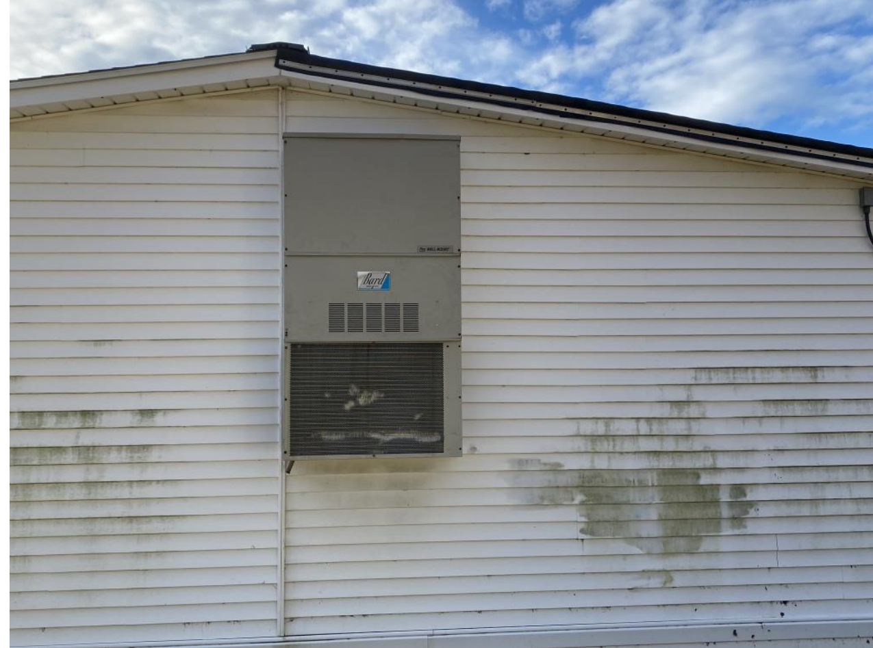
Decaying 20 year old Modulars
