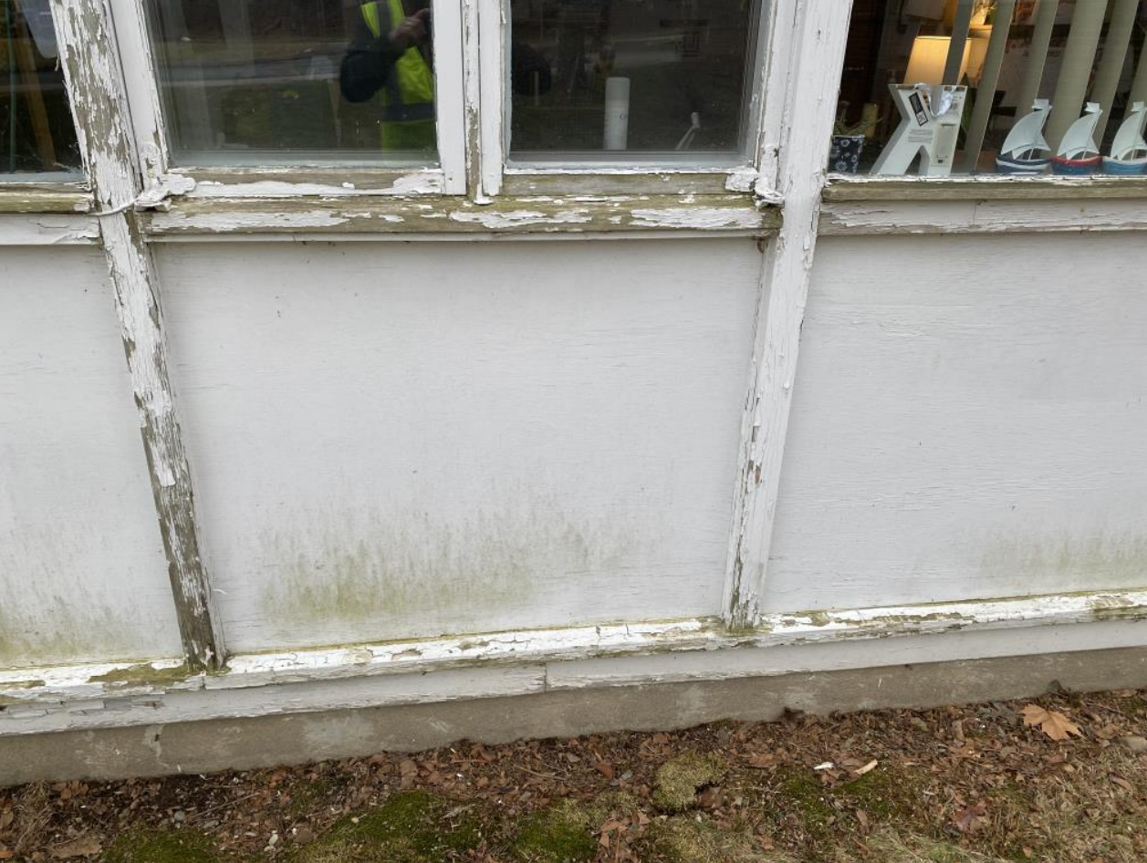
Peeling, rotted wood windows, poor insulation
