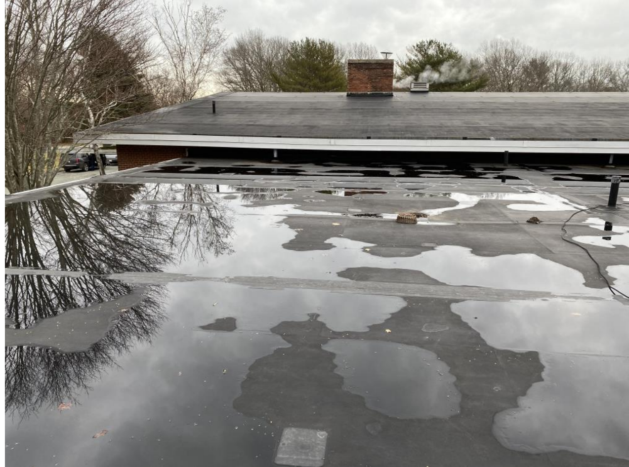
Inadequate roof pitch, leaks
