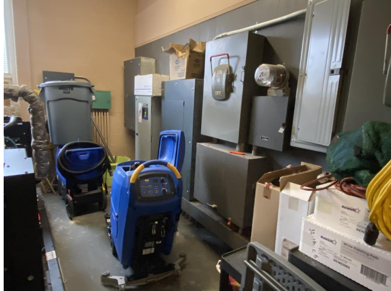
Original 1960's Electrical Switchgear
