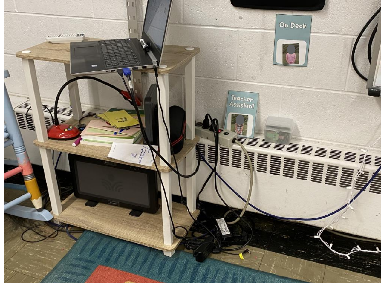
Insufficient Electrical Outlets
