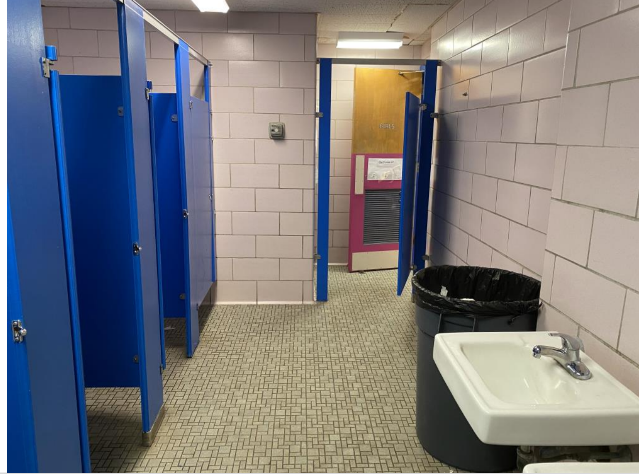
Accessibility at toilet rooms
