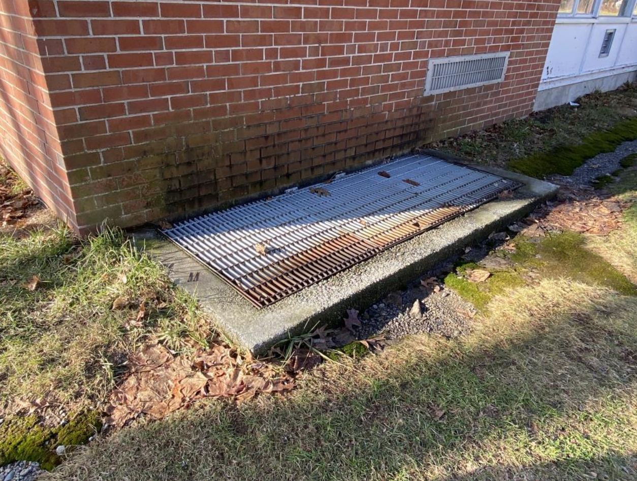
Moisture issues at brick, poor insulation
