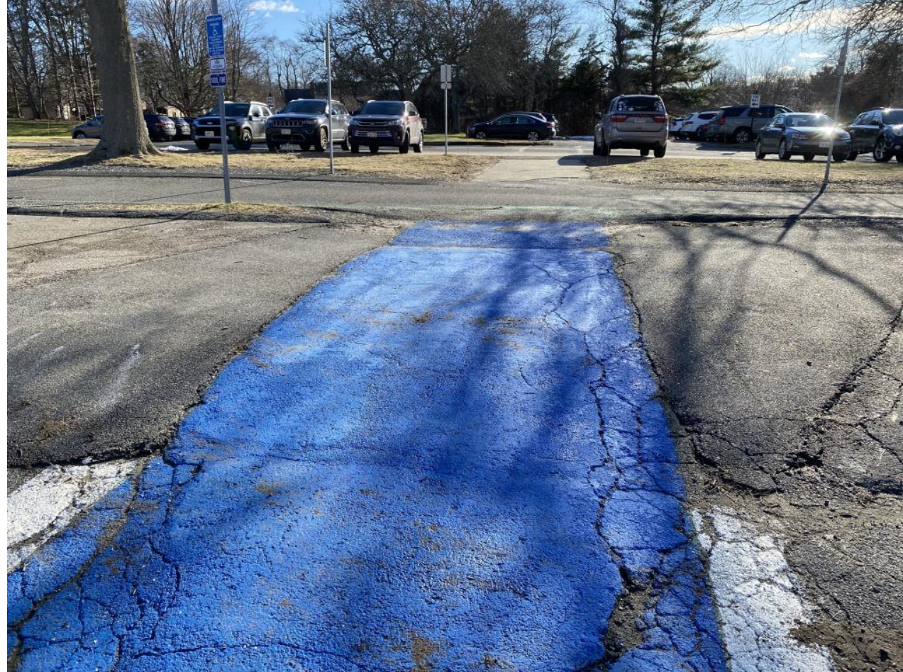
Poor pavement condition, poor site circulation
