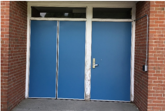
H4. Existing exterior door frames are constructed of wood and have deteriorated beyond usefulness.
