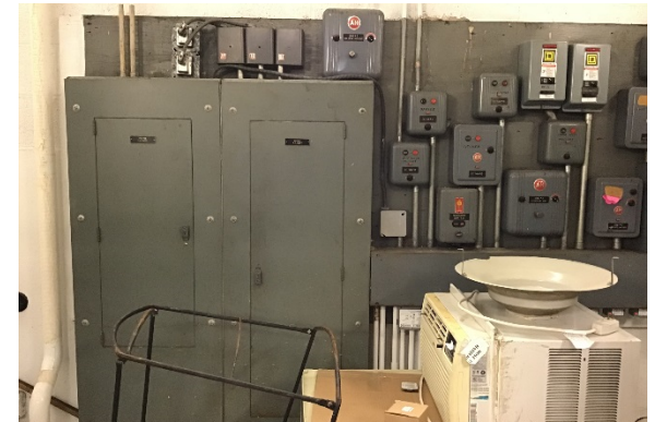
H12. Electrical distribution panels and other equipment are obsolete and should be removed and replaced.
