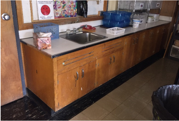
H7. Cabinetry is worn and should be replaced.
