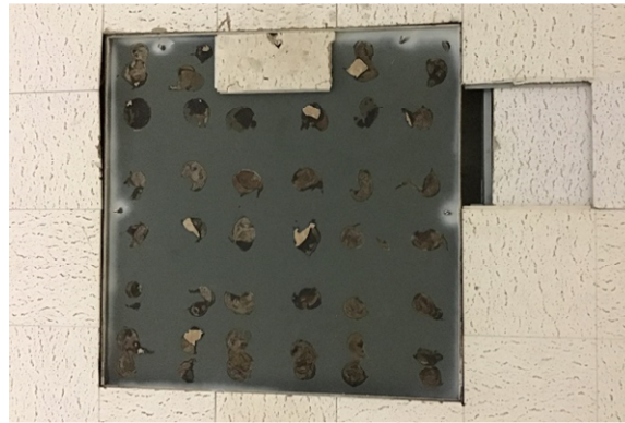
C11. Ceilings are badly damaged and need to be repaired or replaced.
