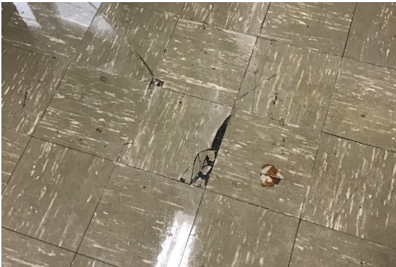
C10. There is 9"x9" floor tile containing asbestos throughout a number of areas in the building.
