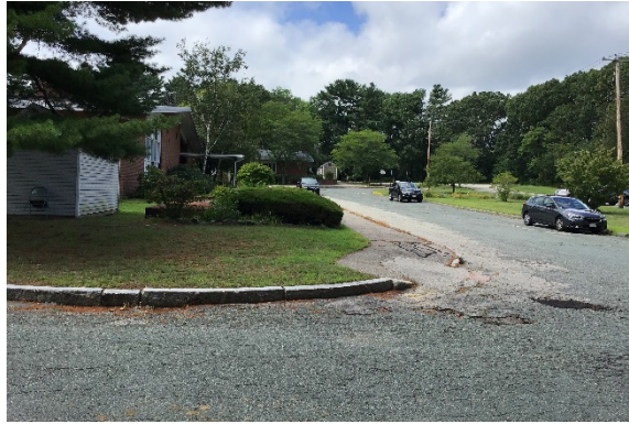
C2. Bituminous paving in the driveway, walkways, and parking area has exceeded its useful life.
