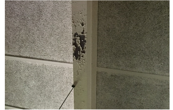
C9. Paint has failed, revealing rust at many of the exposed structural elements in the building.
