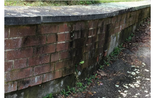
C3. Brick retaining and site walls lack railings as required by code. Masonry is in need of repair.
