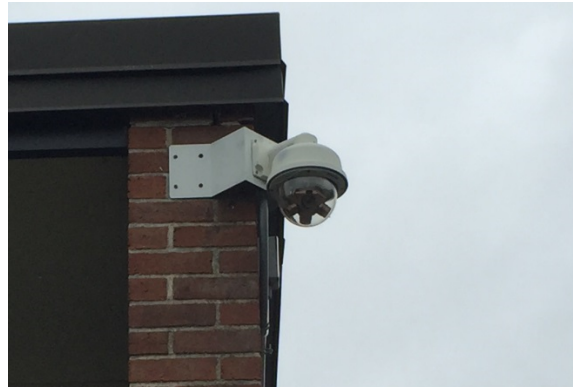
W5. Security cameras are present, but coverage is not presently adequate.
