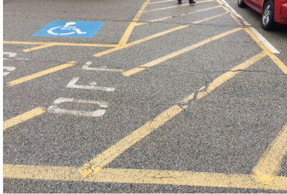
W2. Parking area striping is worn and should be restriped.
