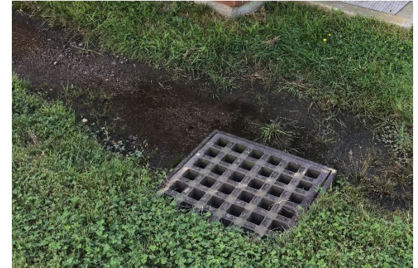
H3. Drainage swales have eroded. Ponding is evident.
