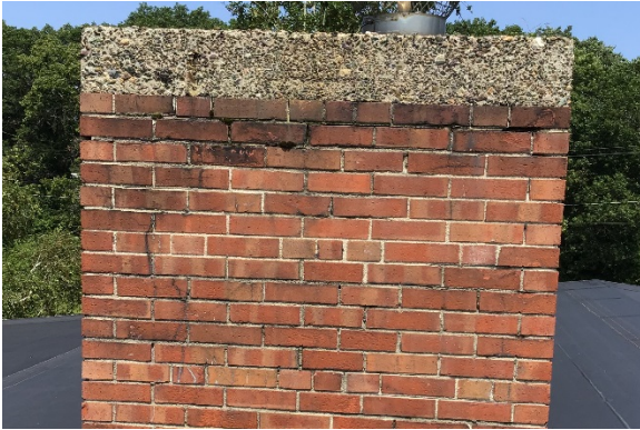
C7. Chimney is badly cracked and mortar has failed. It requires repair and repointing to ensure safety.
