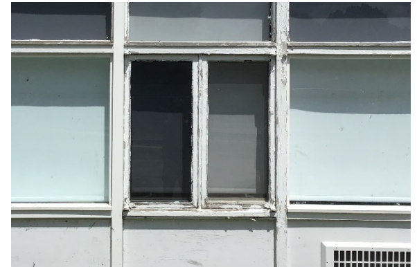
C6. Typical existing windows, hardware, trim, and framing are in poor condition and are not energy efficient.
