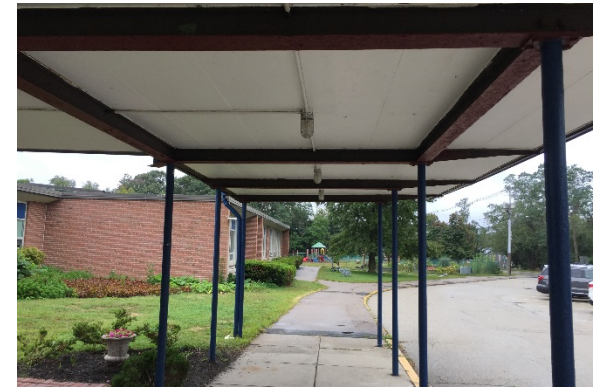
W6. Canopy structural columns and beams are rusting significantly.
