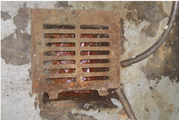
W10. Boiler room floor drain is clogged requiring cleaning or replacement.
