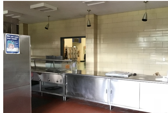
H11. Existing commercial kitchen finishes and equipment need replacement.
