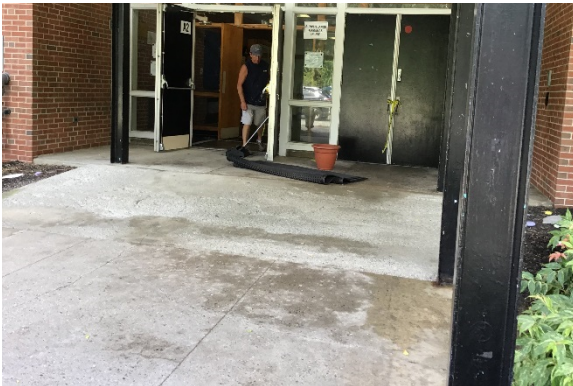
C4. Damaged concrete slabs are uneven and too steep to meet current accessibility codes at all entrances.
