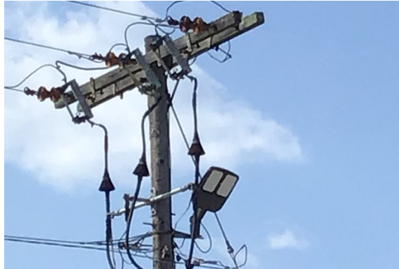
H2. Existing site lighting is inadequate and should be increased.
