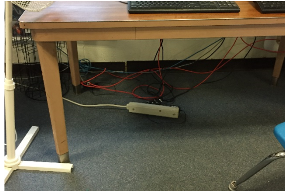
W8. There are currently not enough electrical outlets throughout the building.
