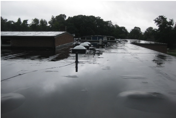
W4. EPDM roof has multiple areas of ponding and delamination. There is an existing leak at the roof hatch.
