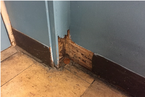
W7. Vinyl base is old and damaged in a number of areas around the building.
