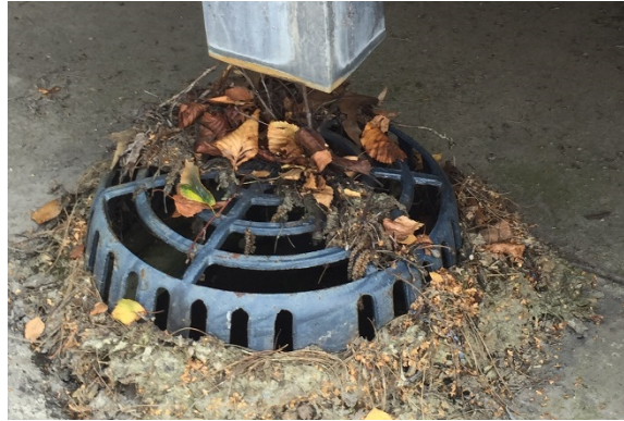
C8. Debris from trees growing too close to the structure make it difficult to keep roof drains clear.
