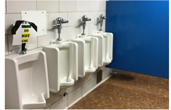
H9. Existing toilet rooms do not meet present plumbing code and should be renovated.
