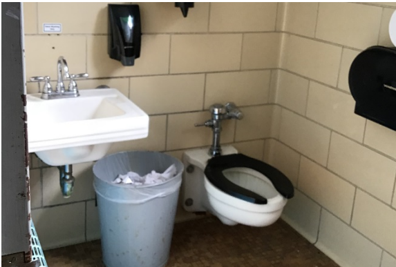
H10. Typical existing toilet room fixtures.
