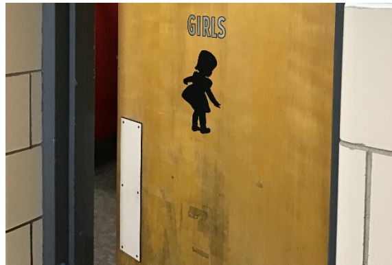
H5. Door signage does not meet ADA requirements and is inconsistent throughout the building.
