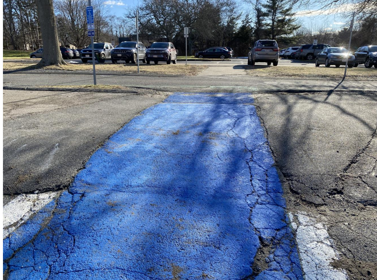
Poor pavement condition, poor site circulation
