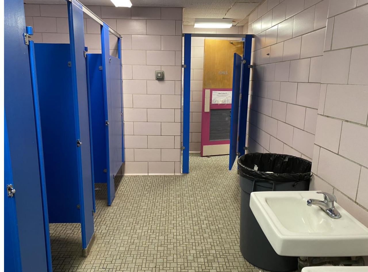
Accessibility at toilet rooms
