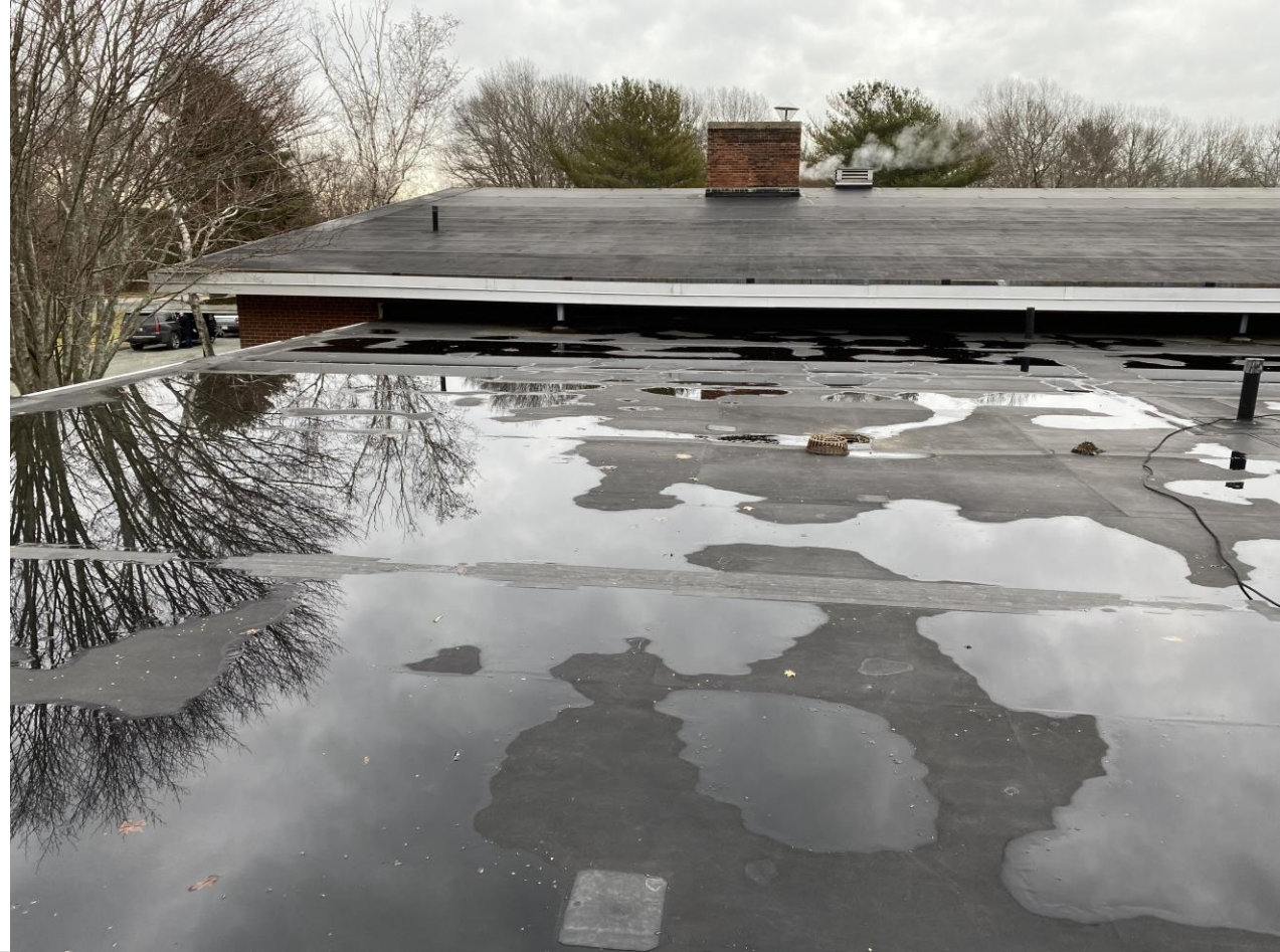
Inadequate roof pitch, leaks
