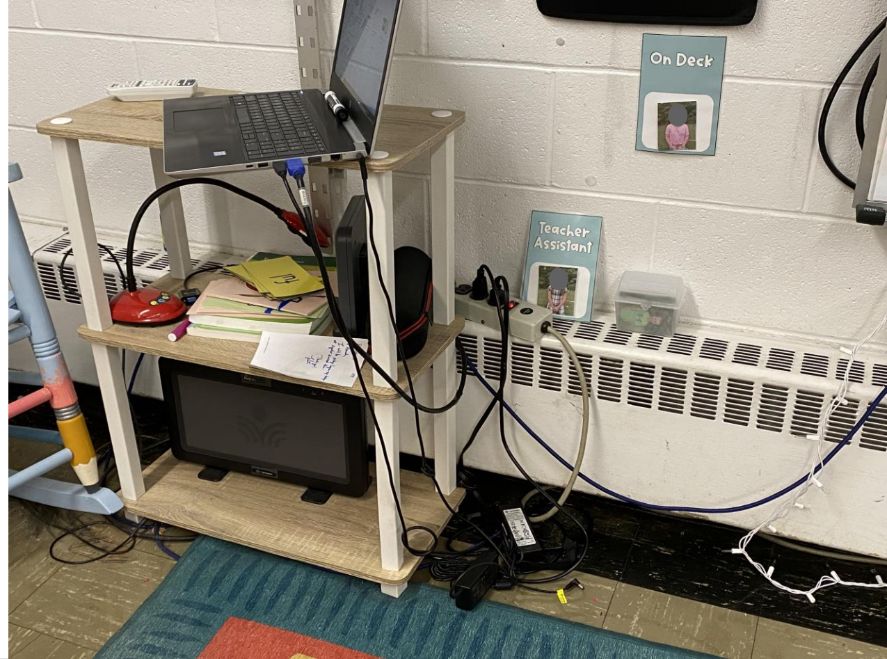
Insufficient Electrical Outlets, power strips used
