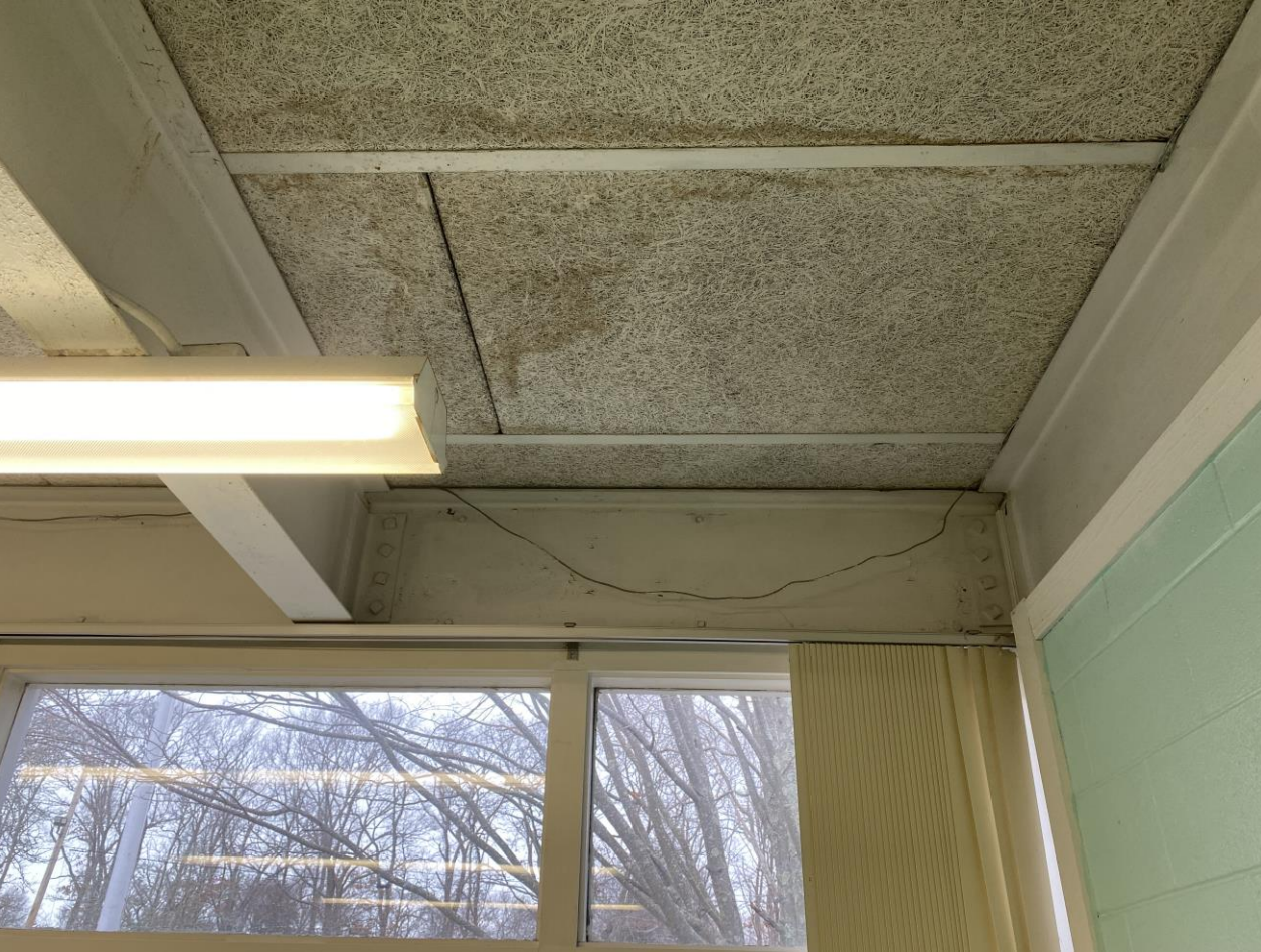
Roof leaks, roof decking not easily repairable
