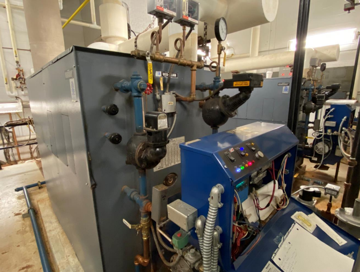
Inefficient, Aging Boilers
