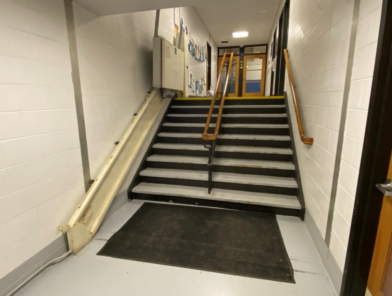
Lift at Stair
