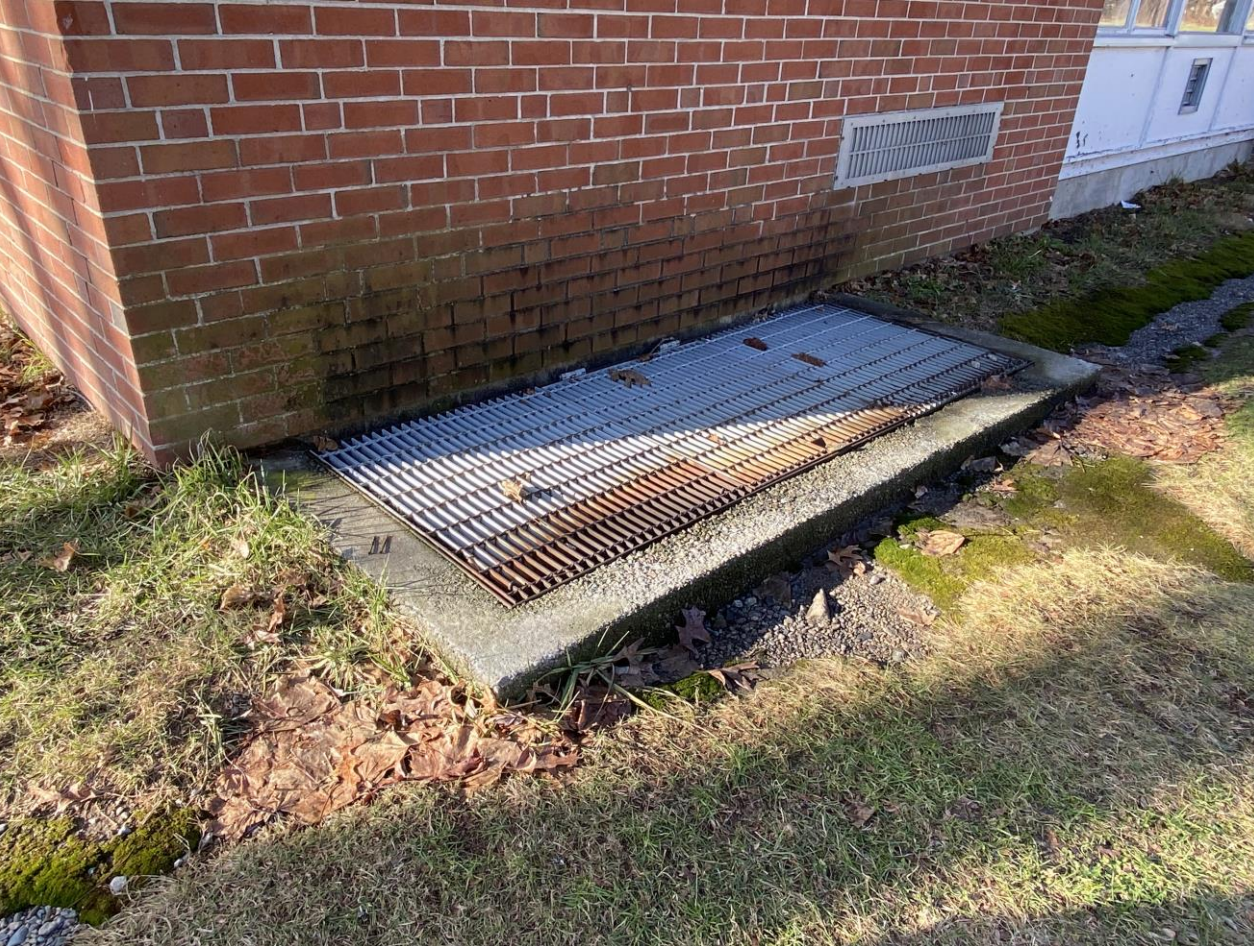
Moisture issues at brick, poor insulation
