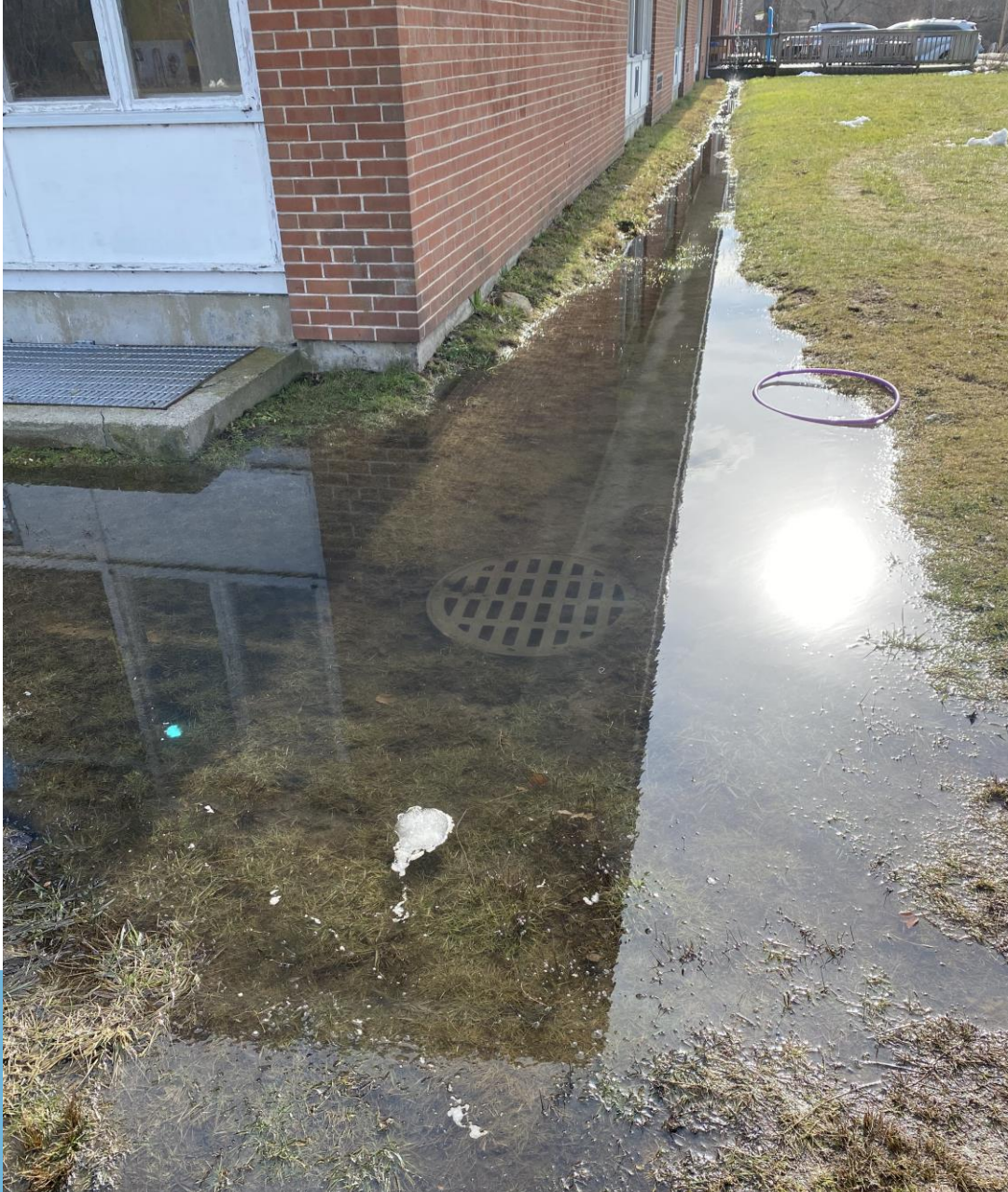
Clogged site drains, poor soil drainage
