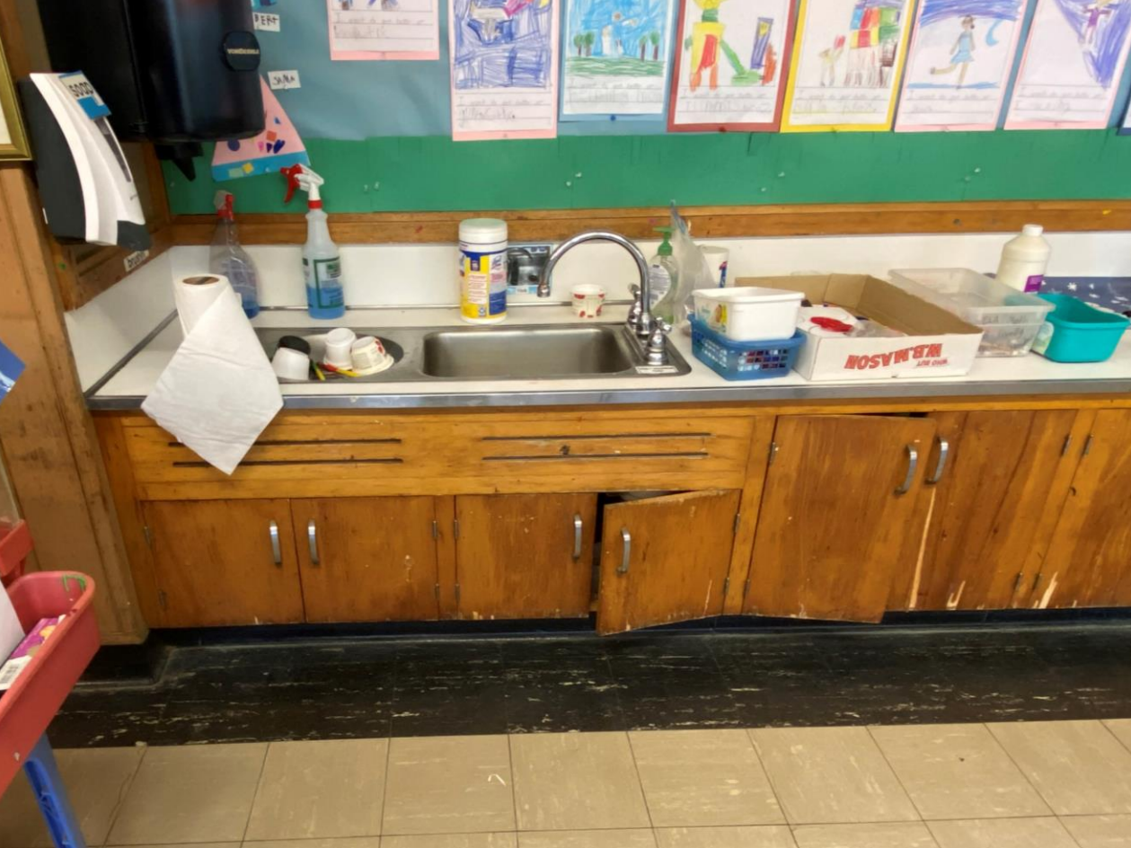
Non-accessible, poor condition classroom sinks
