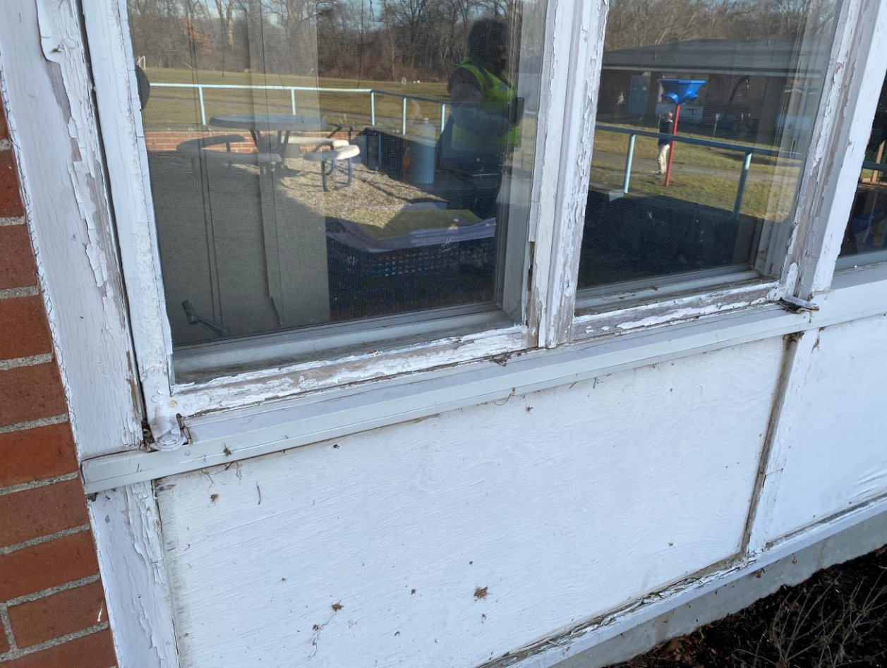
Peeling, rotted wood windows, poor insulation
