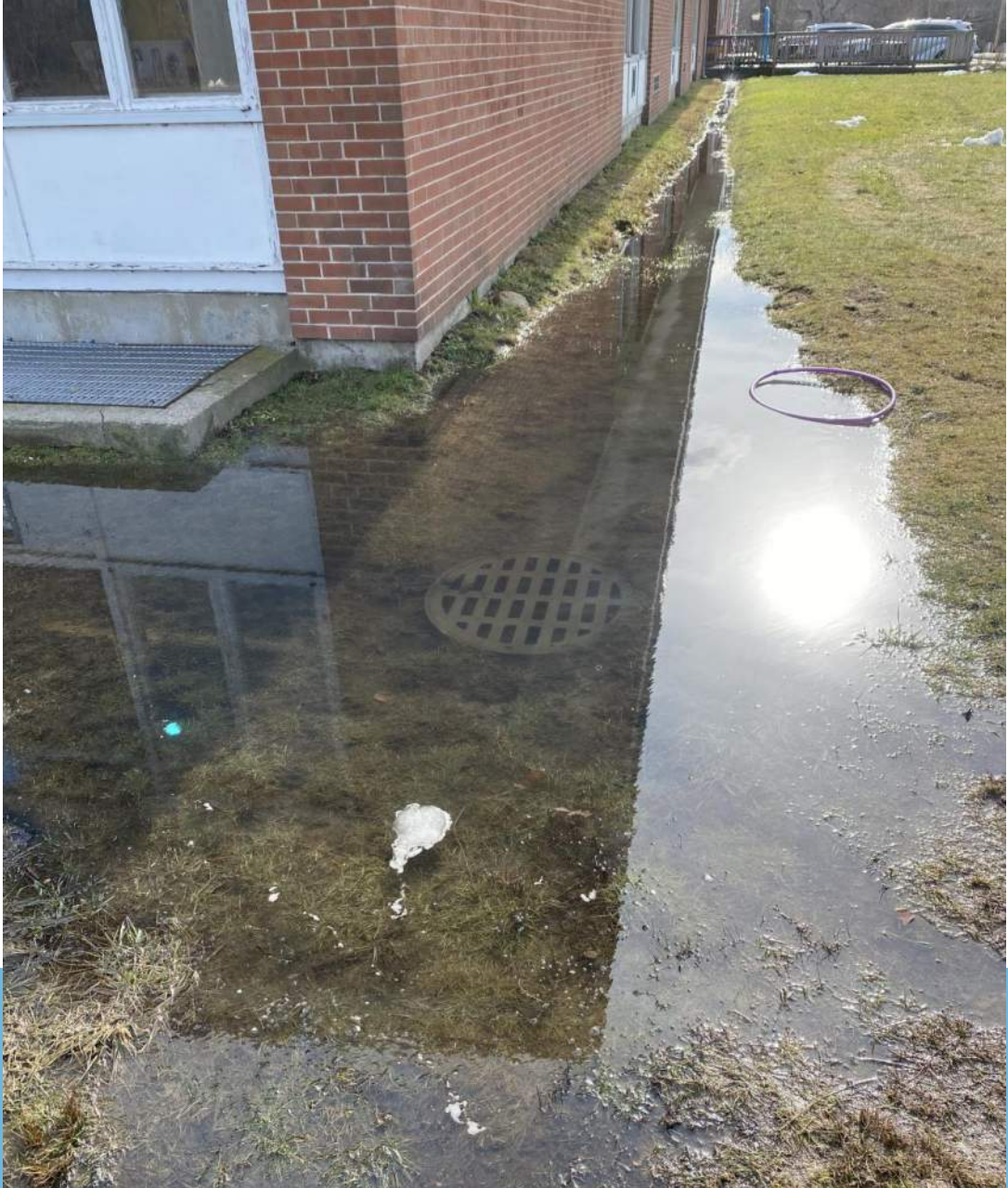
Clogged site drains, poor soil drainage
