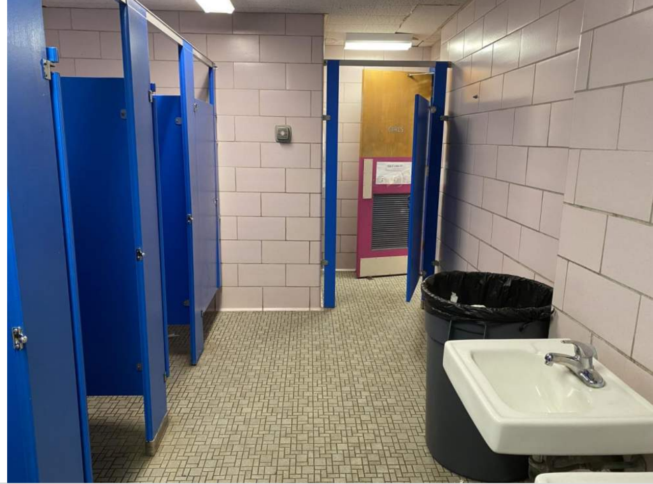
Accessibility at toilet rooms
