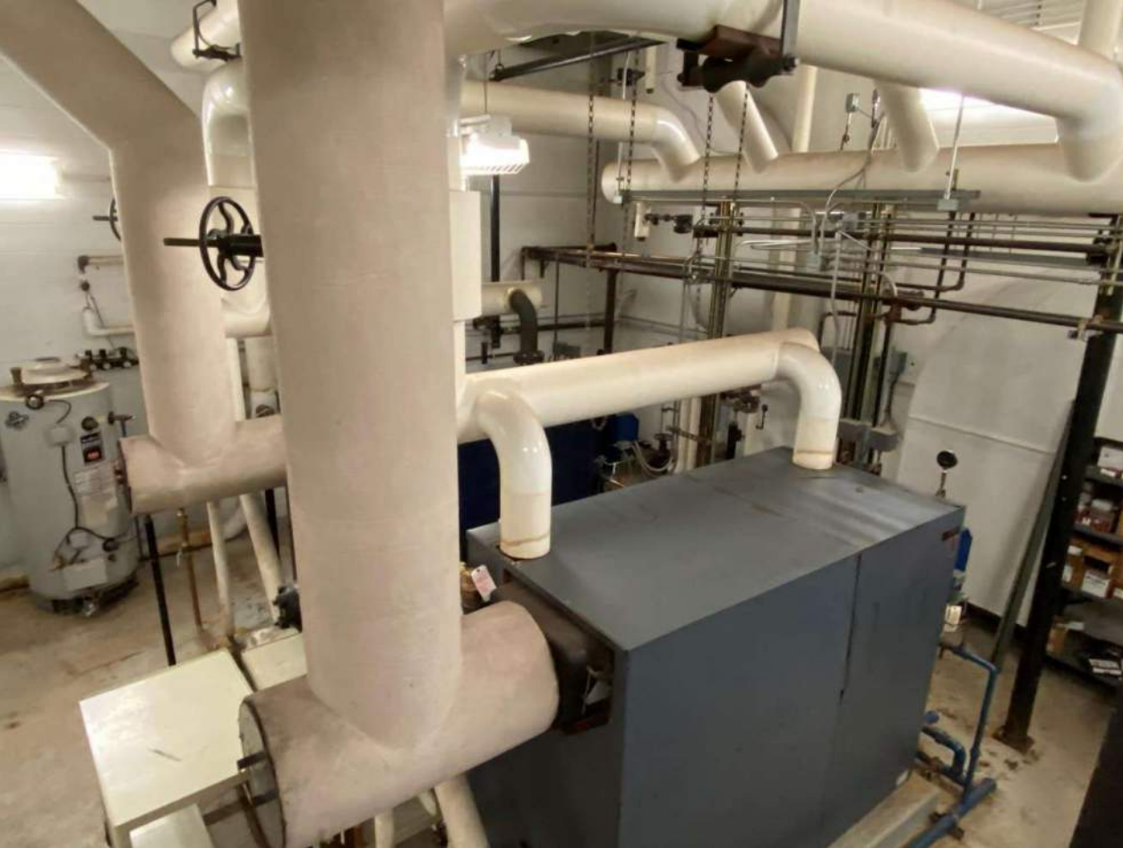
Inefficient, Aging Boilers
