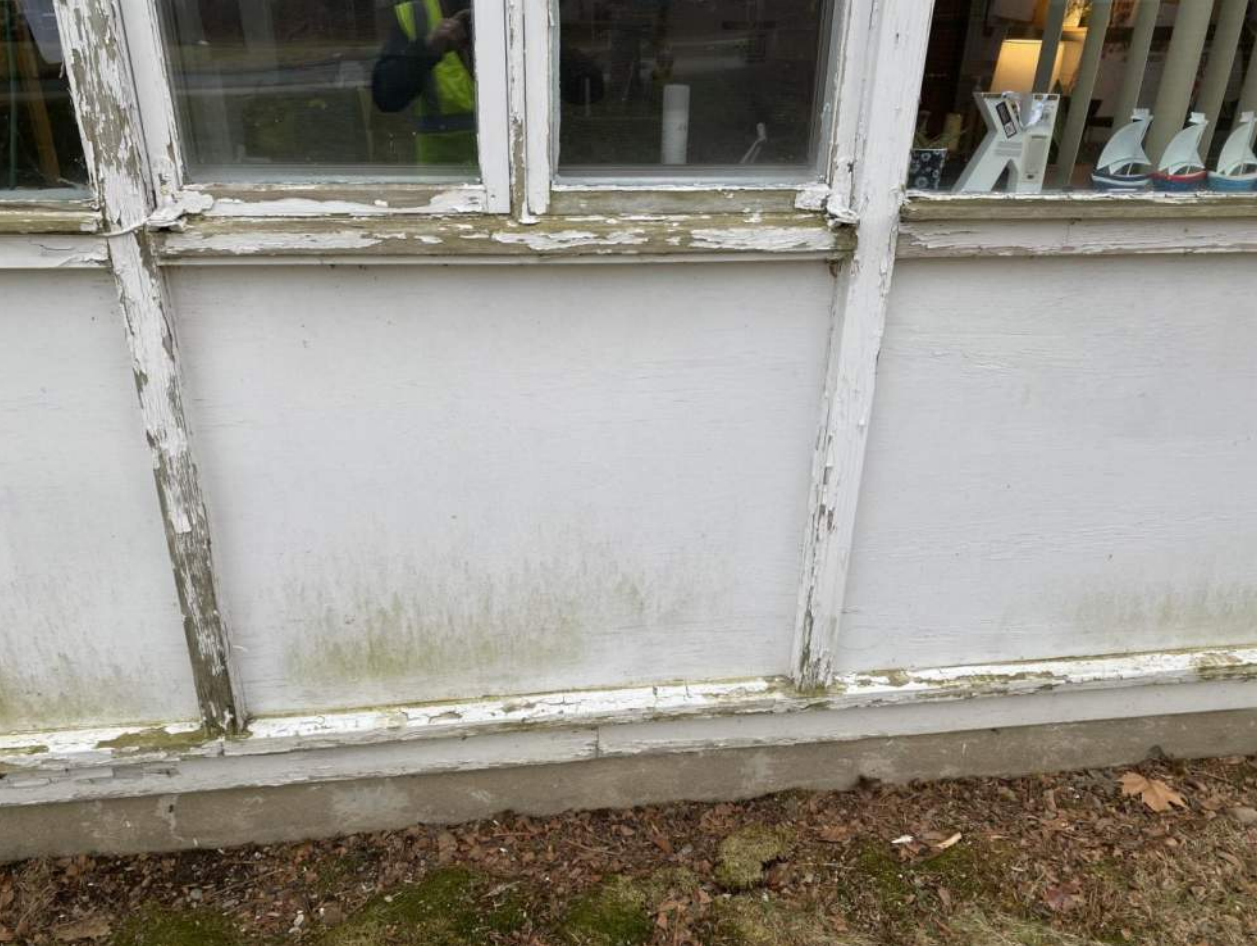
Peeling, rotted wood windows, poor insulation
