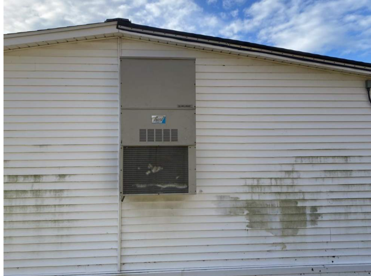
Decaying 20 year old Modulars
