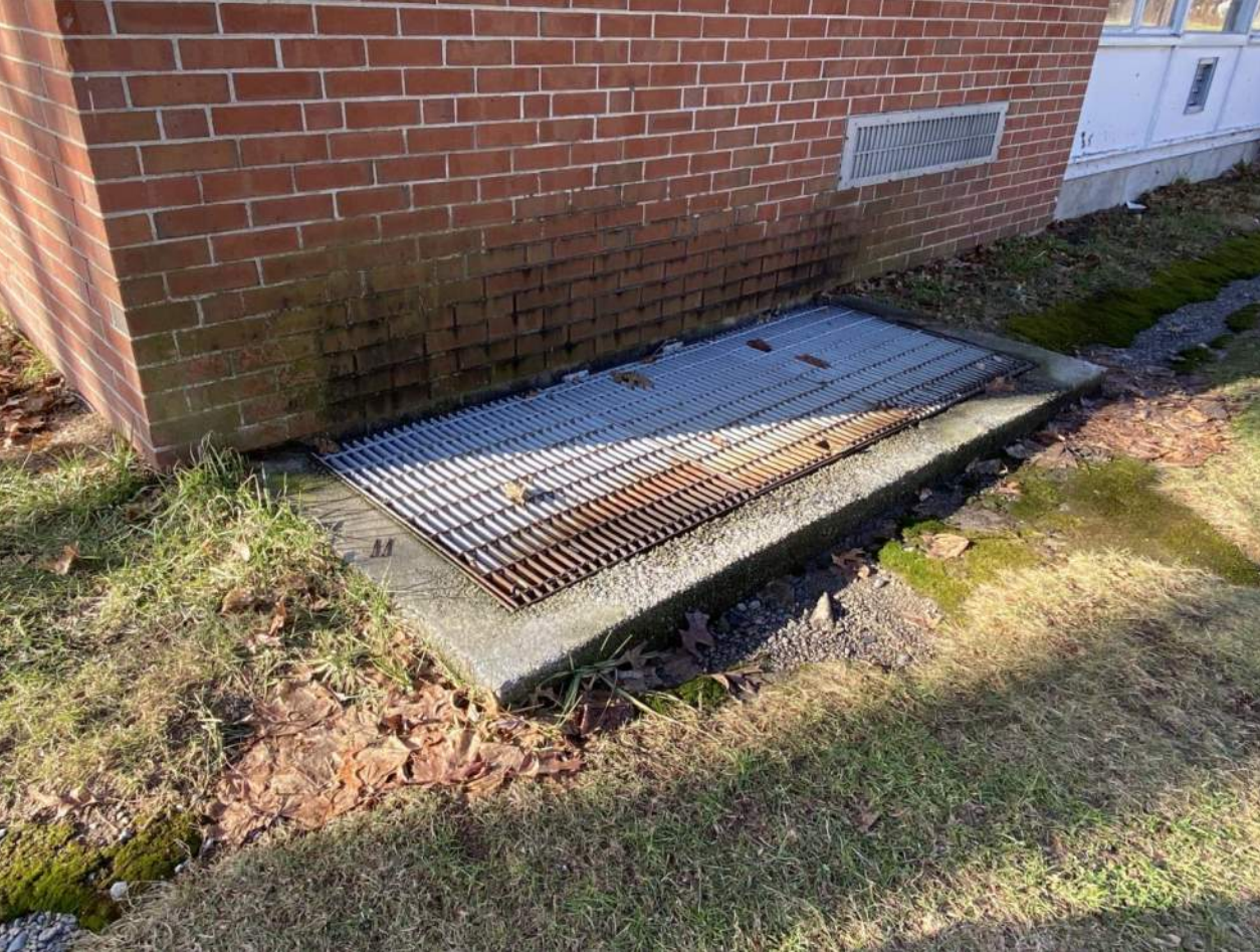
Moisture issues at brick, poor insulation
