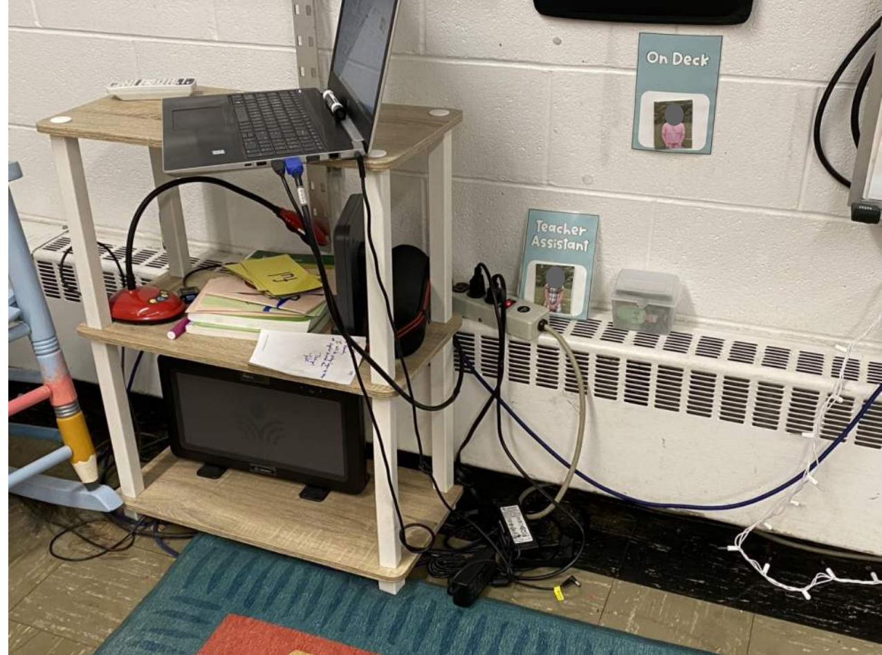
Insufficient Electrical Outlets
