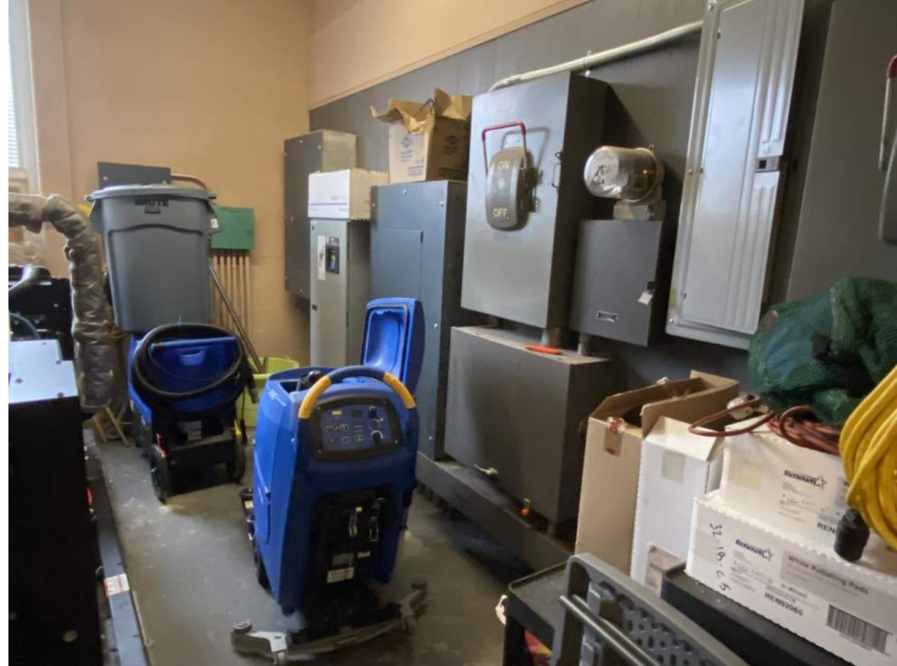
Original 1960's Electrical Switchgear
