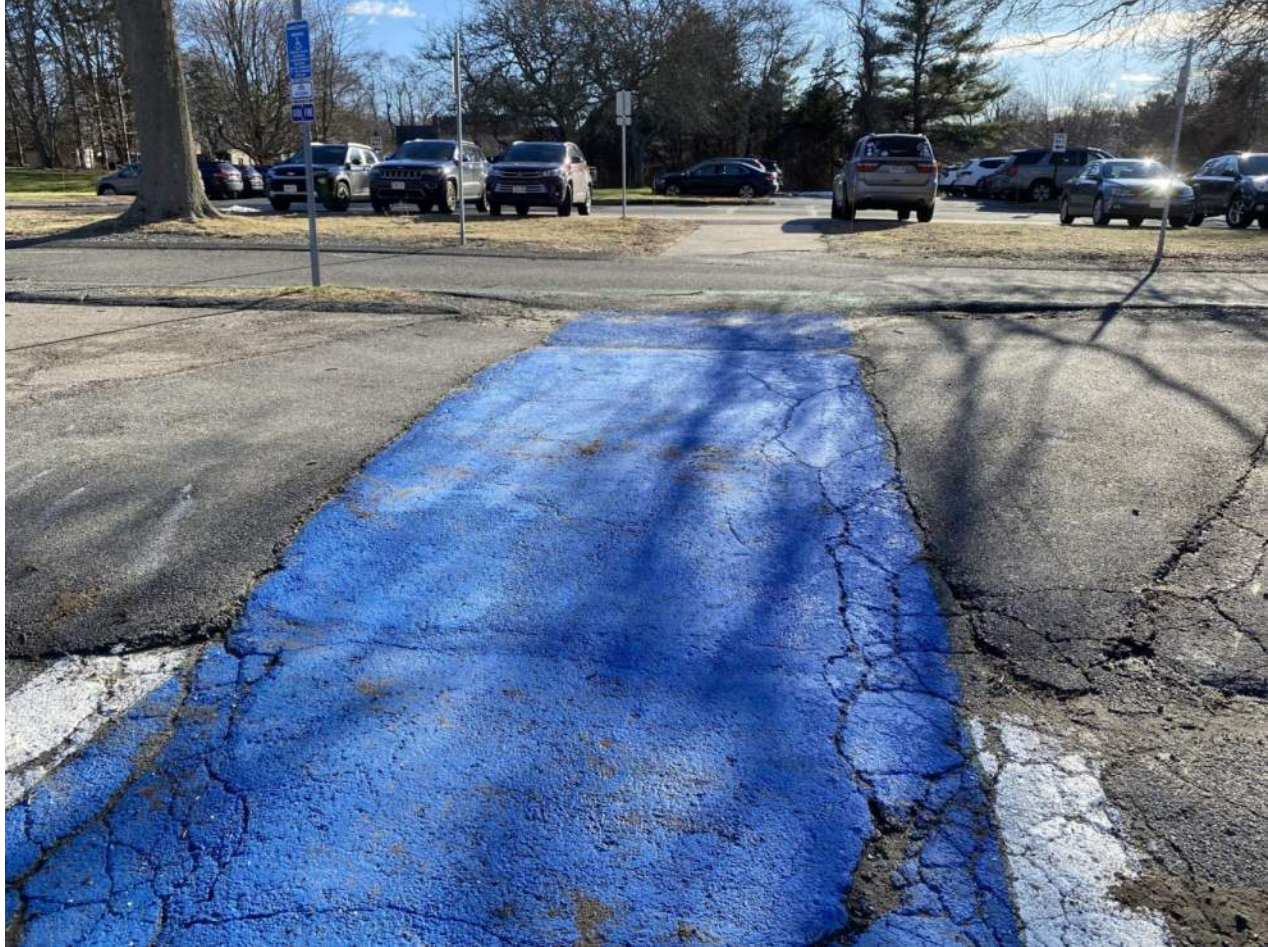
Poor pavement condition, poor site circulation
