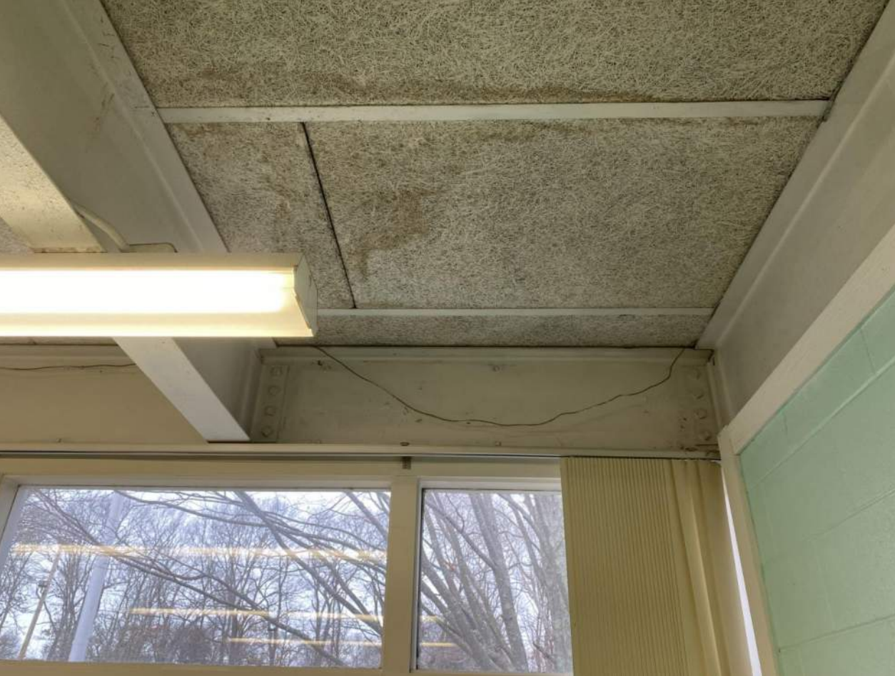
Roof leaks, roof decking not easily repairable
