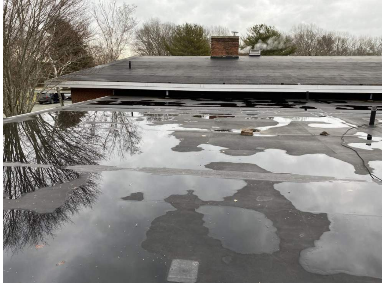
Inadequate roof pitch, leaks
