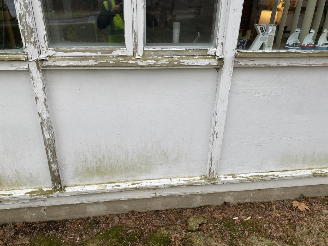
Peeling, rotted wood windows, poor insulation
