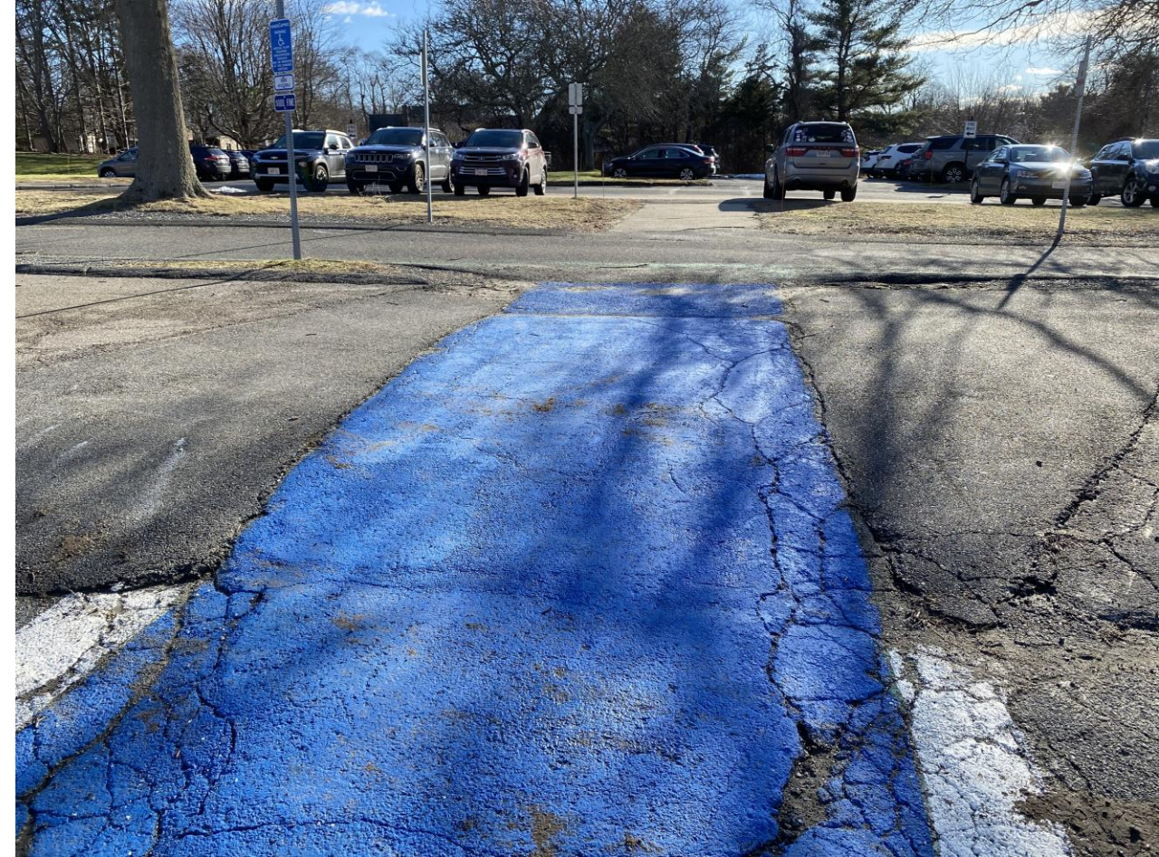
Poor pavement condition, poor site circulation
