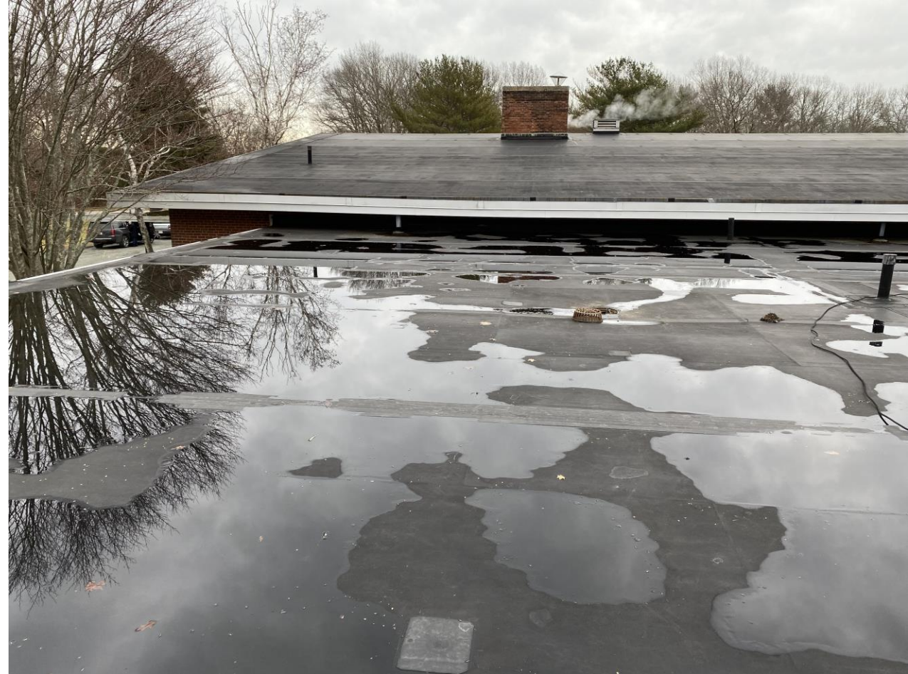
Inadequate roof pitch, leaks
