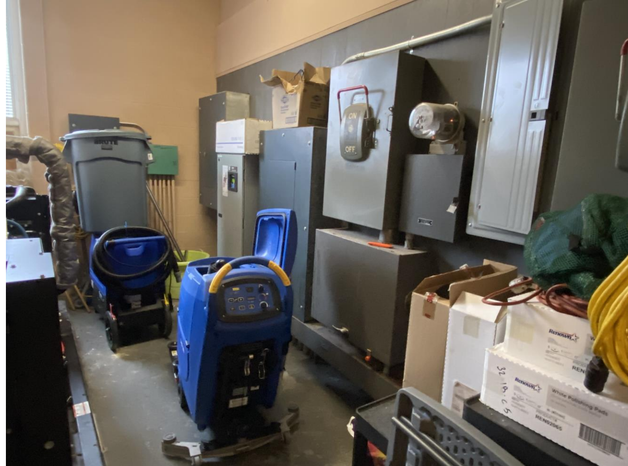
Original 1960's Electrical Switchgear
